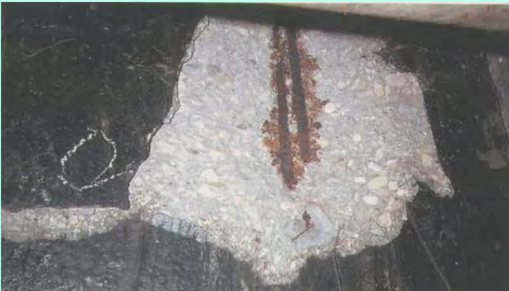
Corrosion of reinforcing bars in the slab
