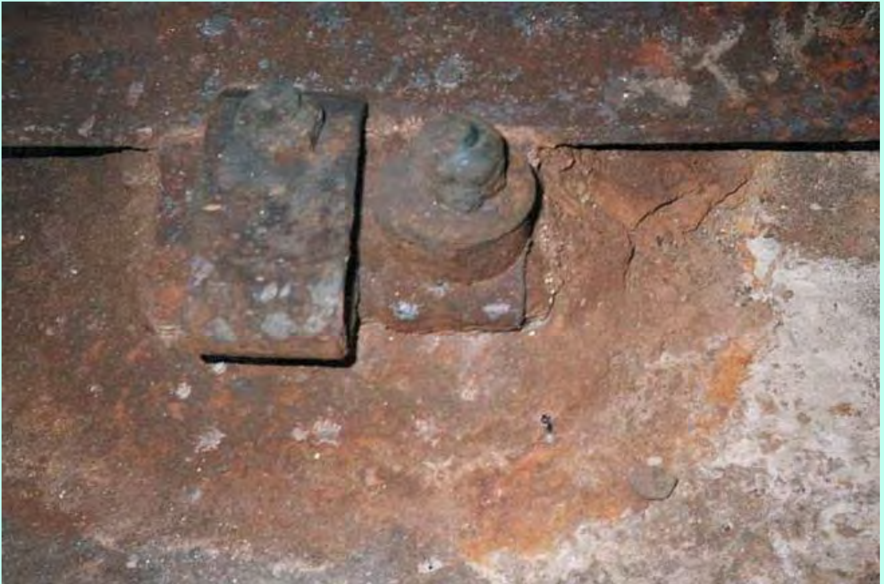
Corrosion of Rail Track due to Leakage
