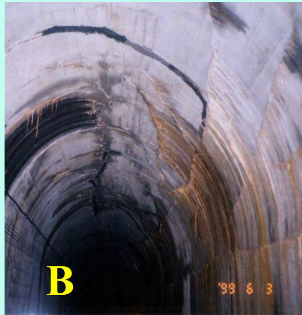
A number of cracks
