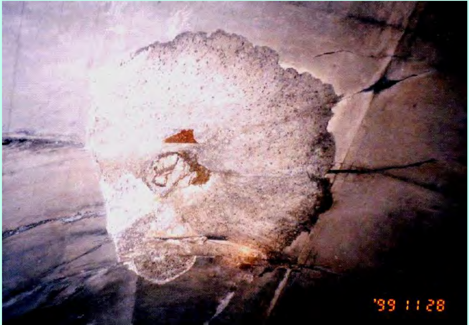
Lining of C tunnel after spalling
