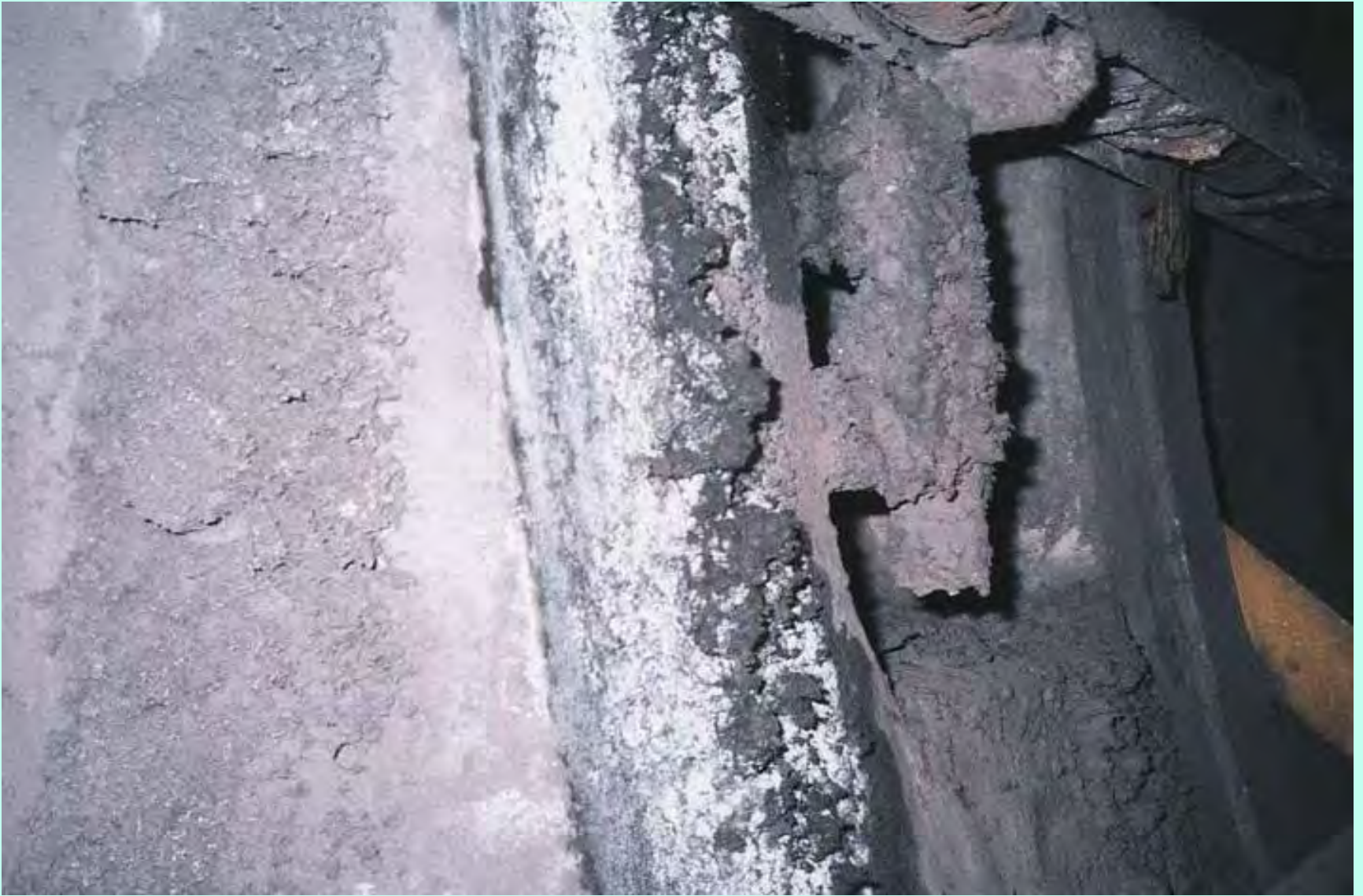
Adhesion of Dust due to Leakage
