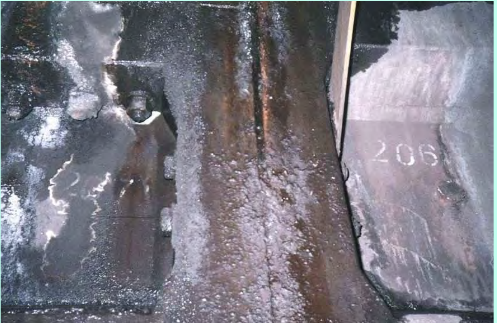
Leakage from Joints of Segmental Lining
