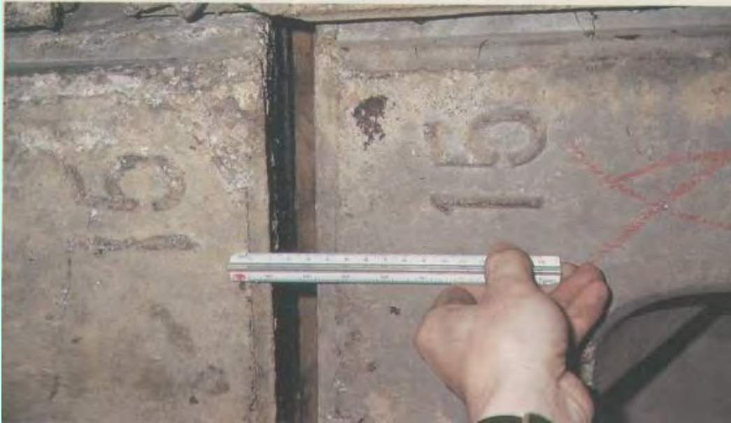
A gap at the joint part of the segment
