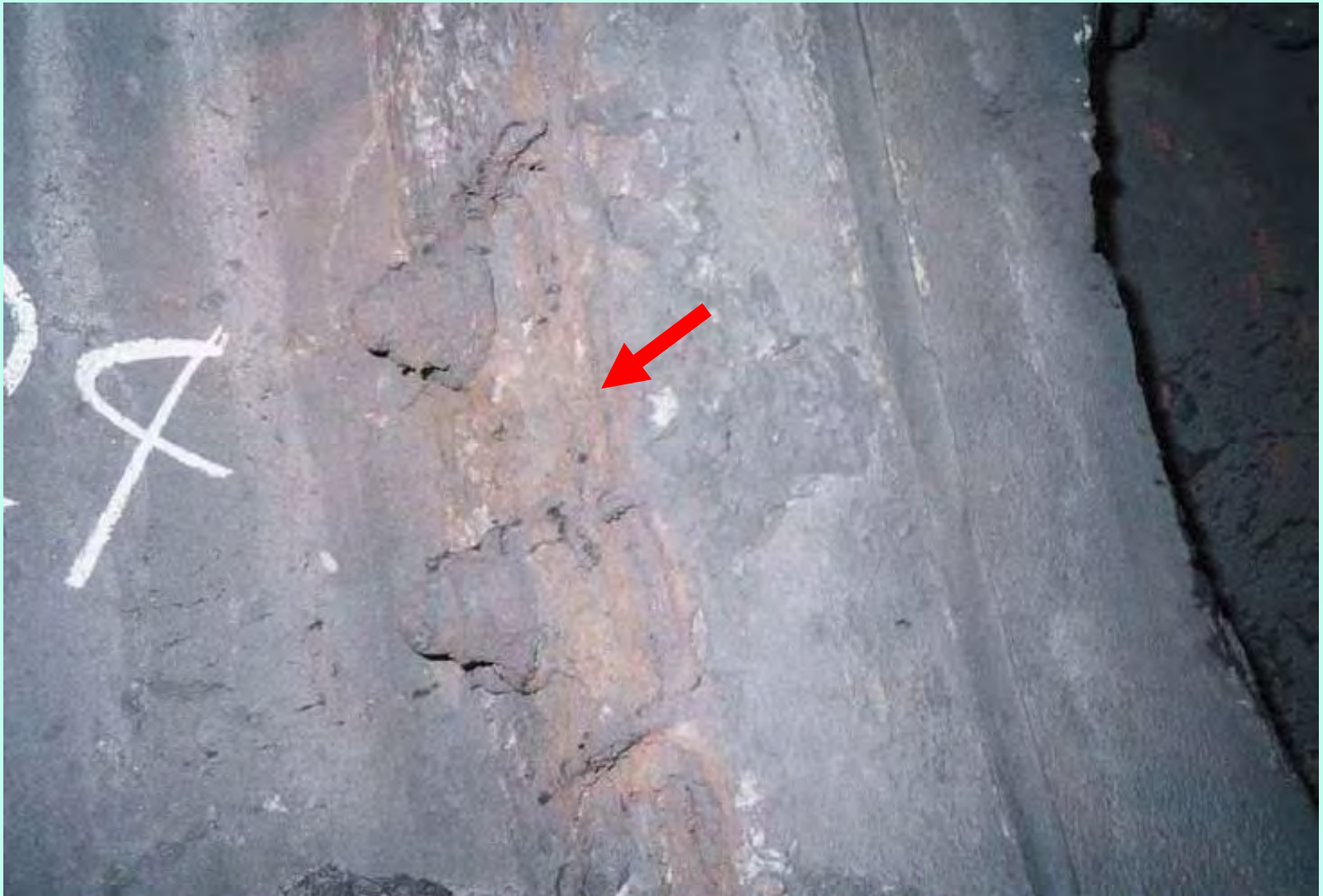
Exposure of Reinforcing Bar due to Lack of Cover Concrete
