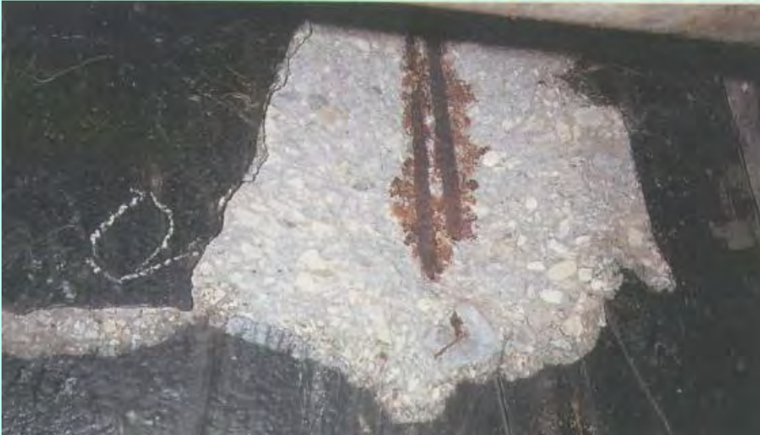
Corrosion of reinforcing bar in the slab
