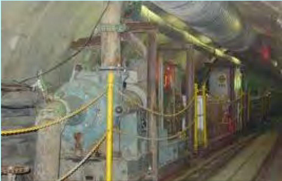
Slurry discharge pump measured to high water pressure (1.5MPa)
