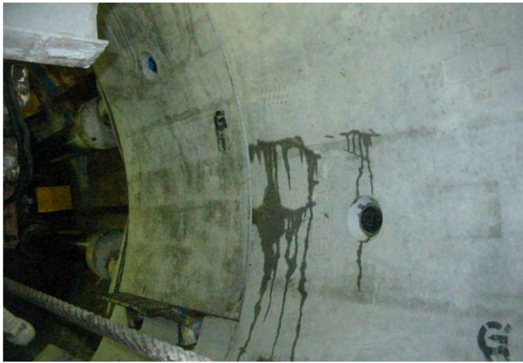
Cracks due to thrust force
